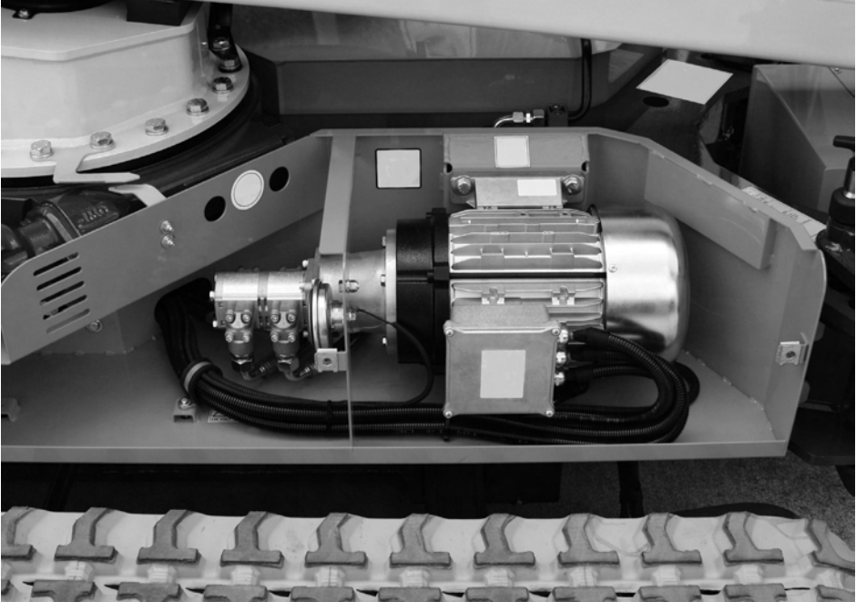
Fig. 168 Electric motor location
