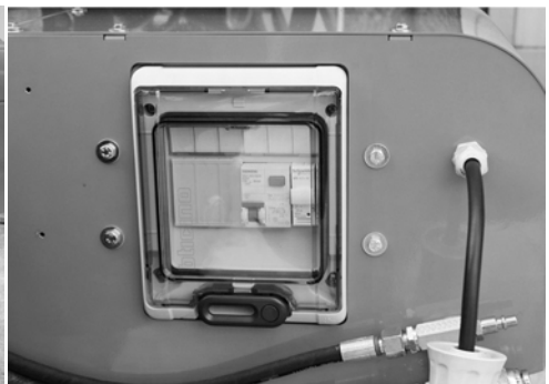
Fig. 87 Main electric switch
